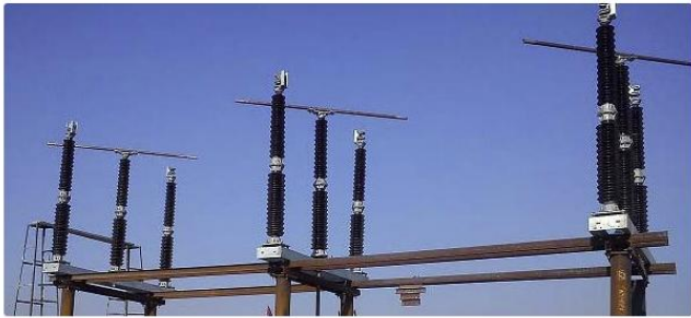
2. Double Break Isolator (DBR).
