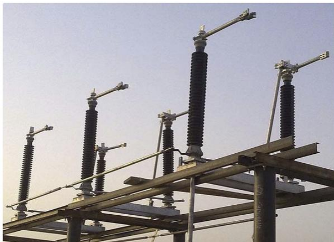
1. Horizontal Centre Break (HCB) Isolator.
